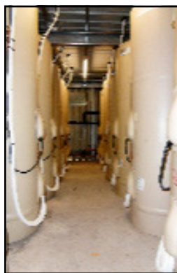
Hot Water Storage Units
